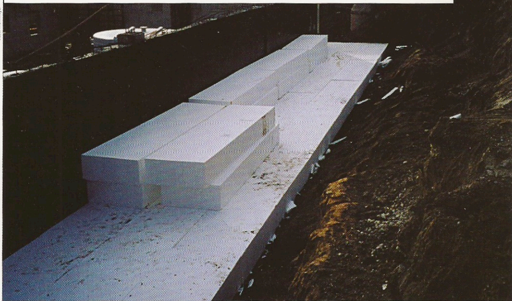
Photo 1: Geofoam backfill at the west wall of microfiltration plant, supporting slab-on-grade pour and reducing lateral pressure on foundation wall.
