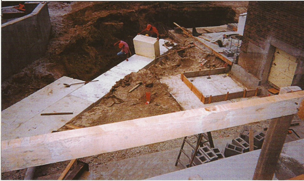
Photo 2: The Manitowoc, Wisc., YMCA uses a footing design similar to the microfiltration plant; here, blocks are placed for spread footing and the elevator shaft.
